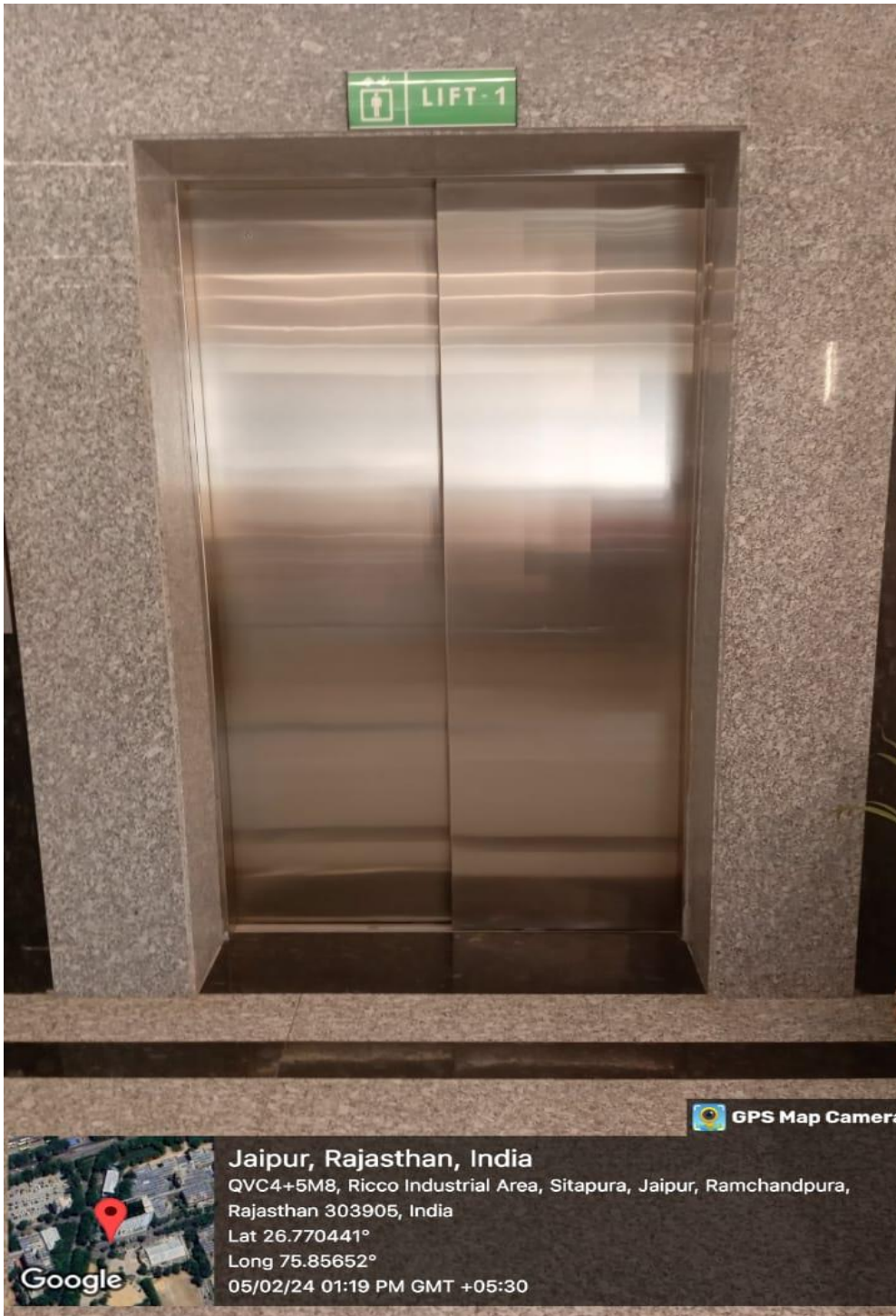
LIFT IN ADMINISTRATIVE BUILDING (RK BLOCK)
